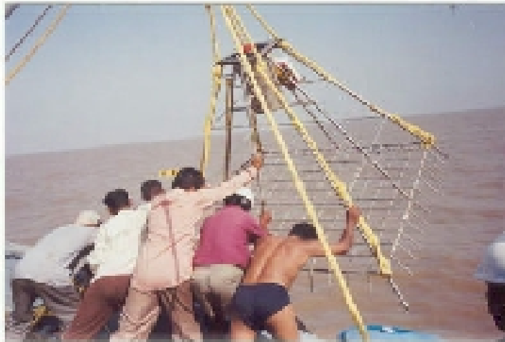
Plate showing the Mooring Frame
