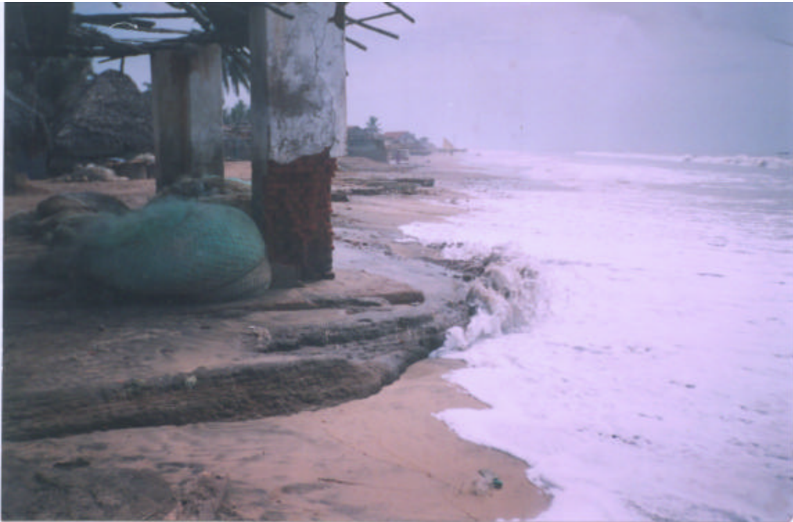
PHOTO SHOWS THE EFFECT OF SEA WAVES ATTACK ON COASTAL STRUCTURES
