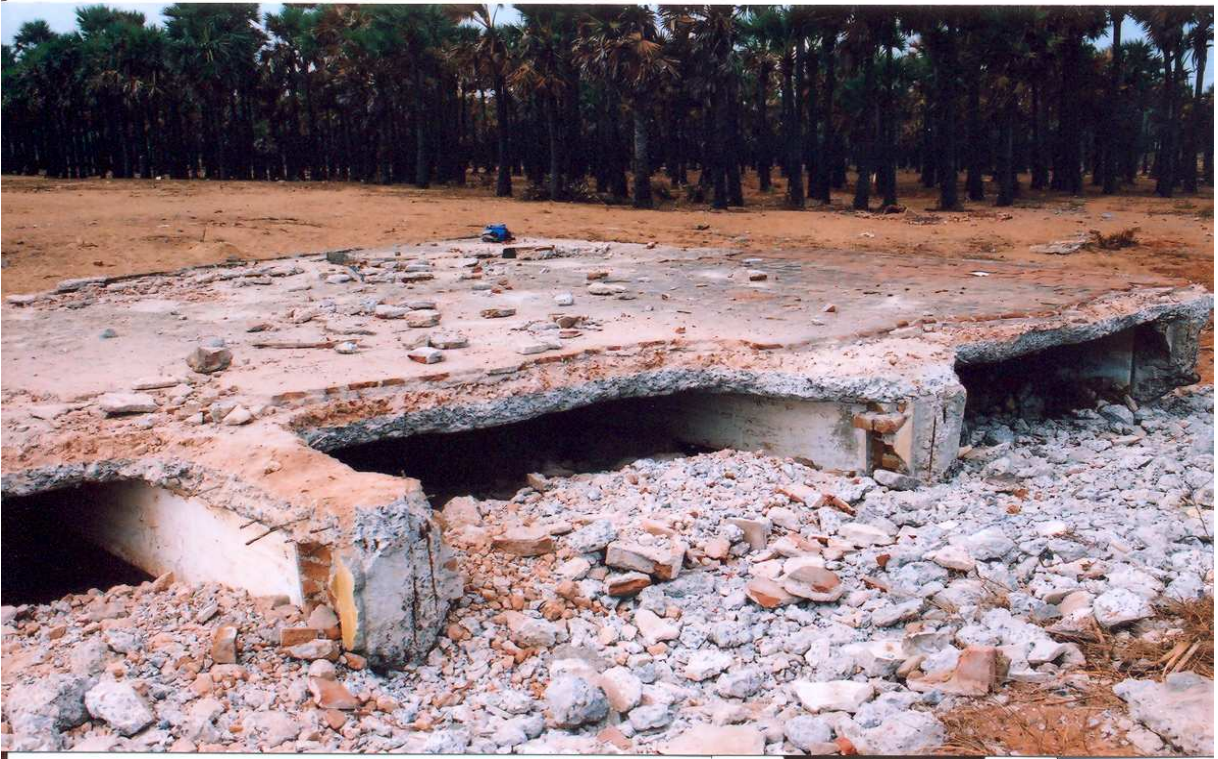
Plate 19. Failed concrete structure (Roof) built with poor quality construction practices (Periyakalpet).
