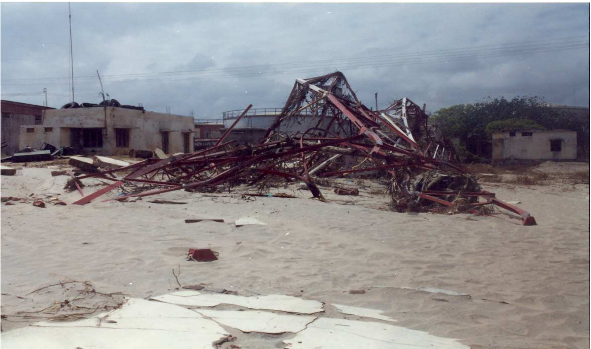
Plate 12. Power transmission tower at Nagapattinam failed by tsunami. The structure is of space-frame type with steel flats and angles
