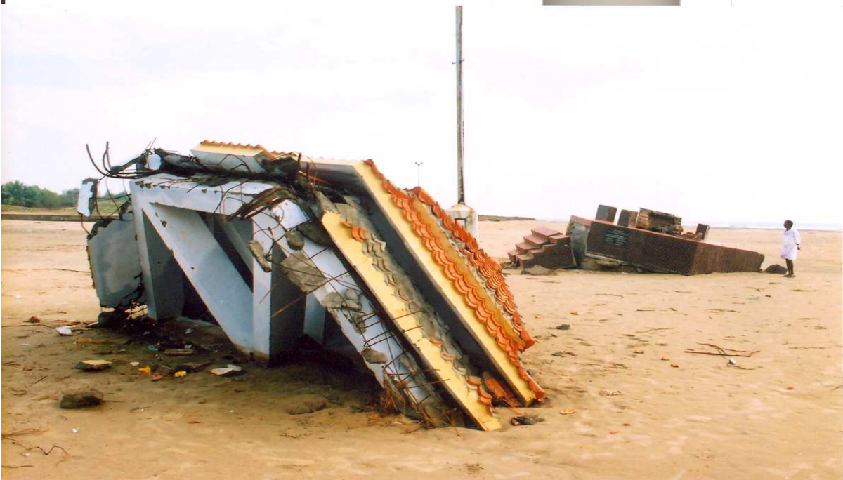
Plate 13. Tsunami damaged reinforced concrete structure on the beach (Cuddalore)
