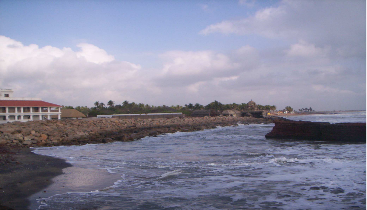
Plate 25. Rubble mound seawall which has considerably reduced the tsunami impact over the structures behind (Tarangambadi).
