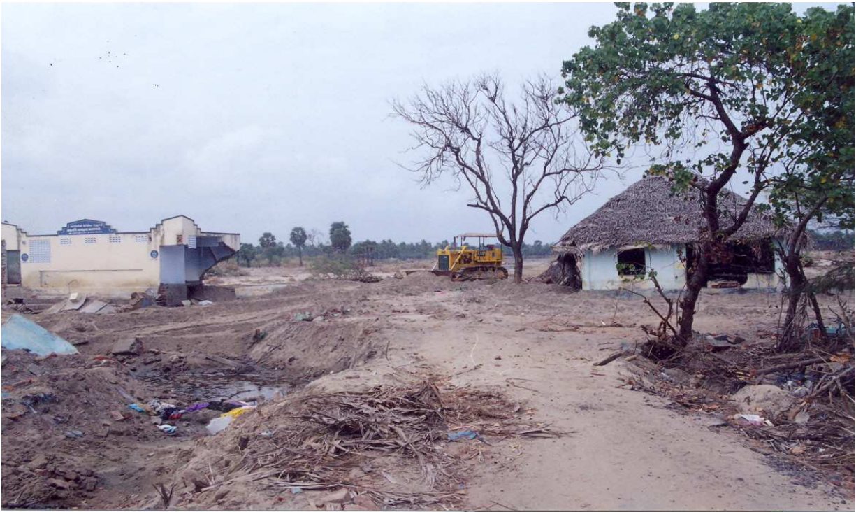
Plate 22. Example of failed structure constructed in lower level (Left) as compared to the unaffected house (right) constructed on higher ground level (Velankanni).
