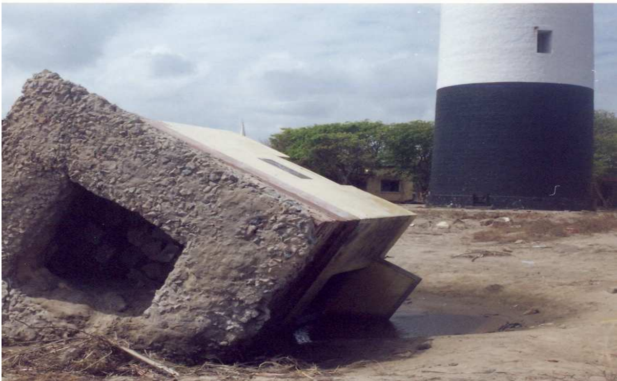
Plate 16. Unaffected light house (circular in plan) at the background and failed structure (rectangular in plan) at the front (Nagapattinam harbour).
