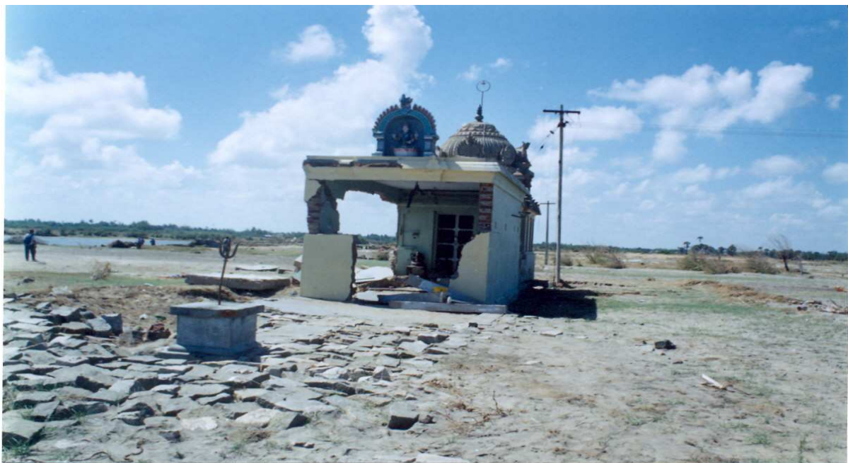
Plate 6. Damaged Cauery temple (Poompuhar) few tens of meters from sea. Isolated and smaller dimensional structures like this are less stable under undiffused tsunami flow due to lesser number of structural members in the lateral dimension.
