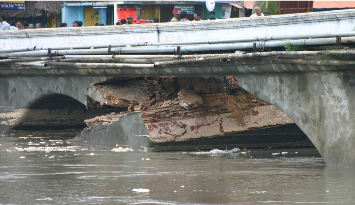
Plate 20. Example of scour failure in one of the piers of very old arched road bridge constructed with brick in lime mortar (Arasalaru river bridge, Karaikal).
