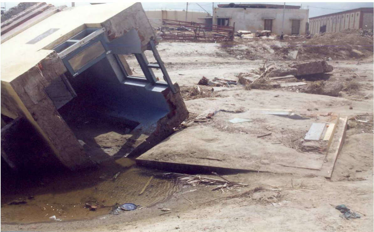
Plate 14. Total failure of isolated and small dimensioned structure in the front and unaffected larger structures in the background (Nagapattinam harbor).
