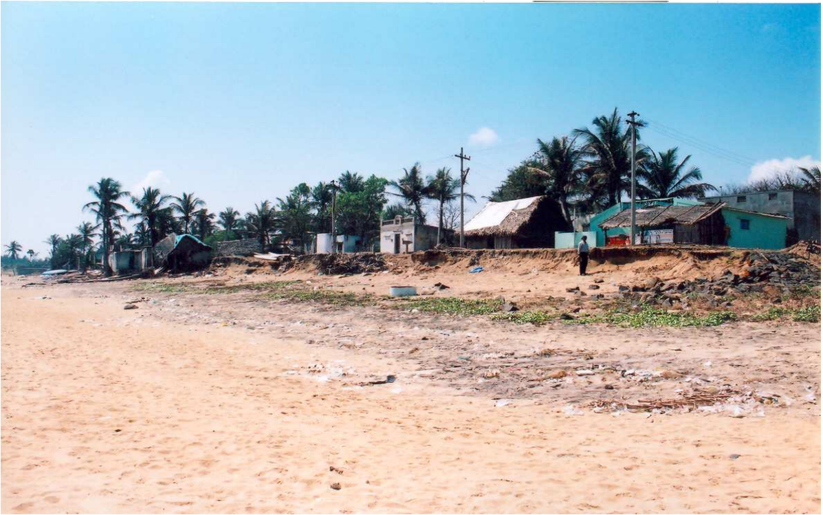
Plate 11. Failure of front row structures built right on the beach few tens of meters away from the sea (Karikattukuppam).
