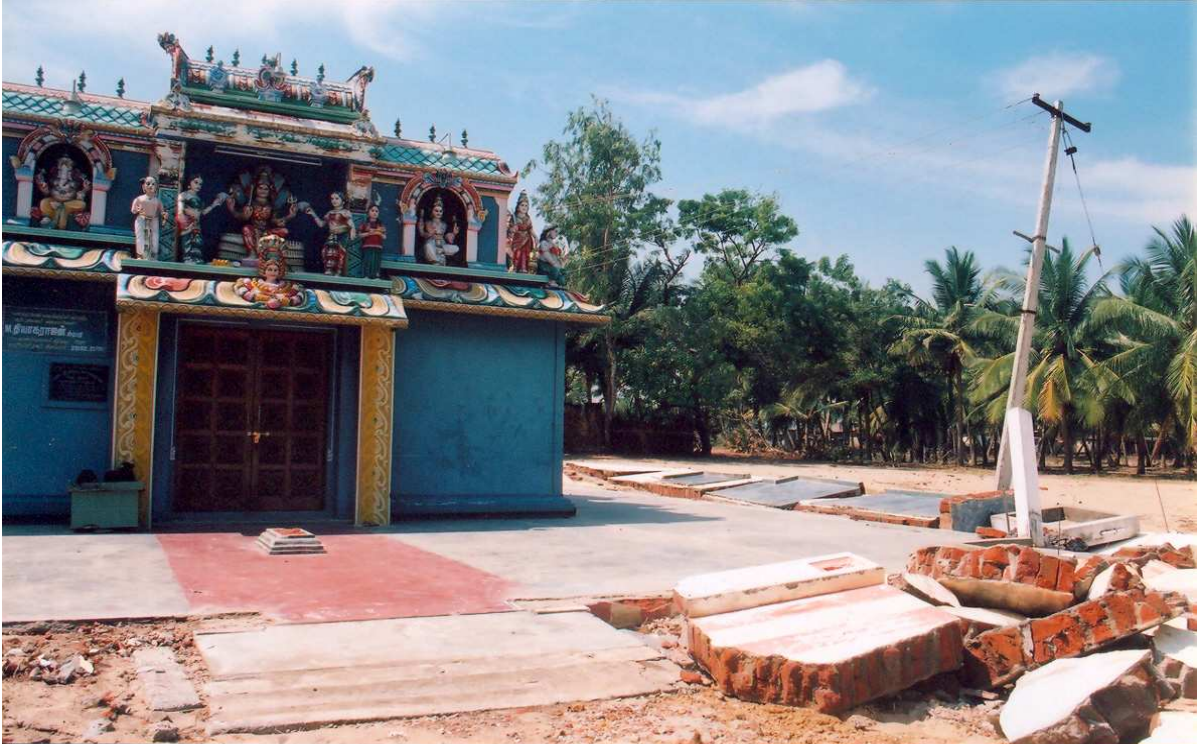
Plate 5. Failure of compound walls. Failures of such non-load bearing short walls are inevitable as they are not designed for lateral impact loads such as tsunami. (Reddiyarpettai)
