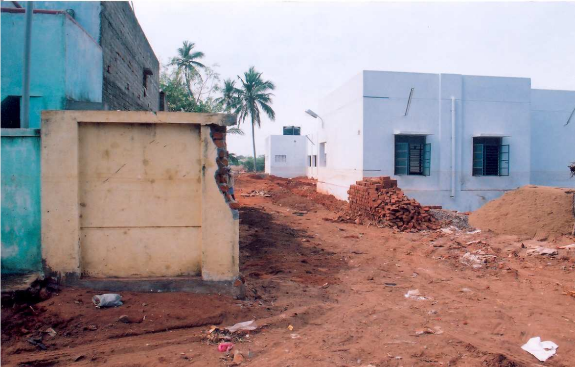
Plate 1. Tsunami water mark on the walls of a building in Periyakalpet. Such marks were used to deduce run-up and inundation limit.
