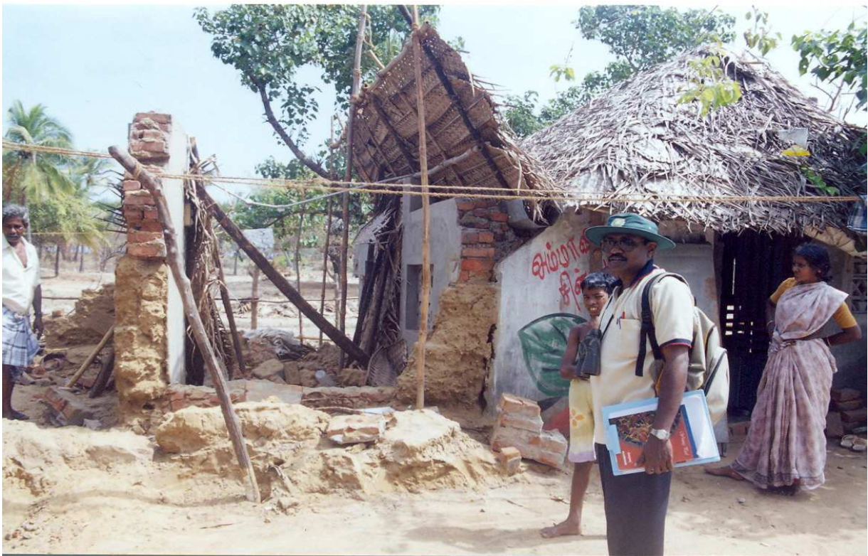
Plate 18. Failed mud plastered brick house (Velankanni).
