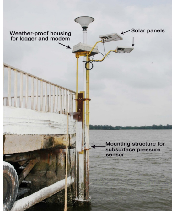
Fig. 1 Typical installation of subsurface pressure sensor based sea level gauge
