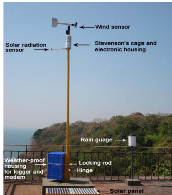
Fig. 3 Typical installation of AWS in NIO's ICON network
