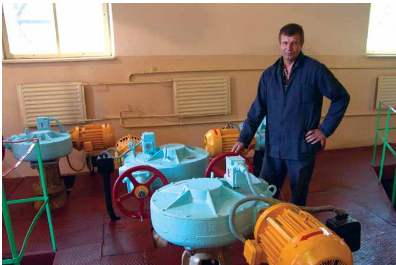
Main sewage pump center in Chernigov, Ukraine
